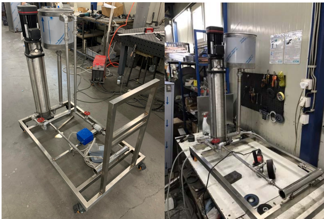
Figure 1 Membrane filtration unit during the upgrade in the production stage
